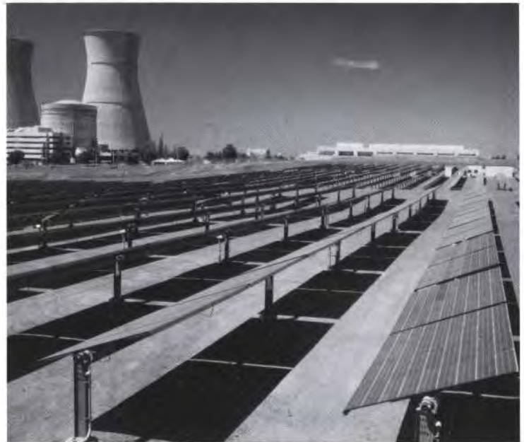
As the cost of photovoltaics continues to decrease, the technology becomes increasingly competitive for utilities. Above is a 2-MW single-axis-tracking photovoltaic system at Sacramento Municipal Utility District's Rancho Seco facility in Sacramento, California.
